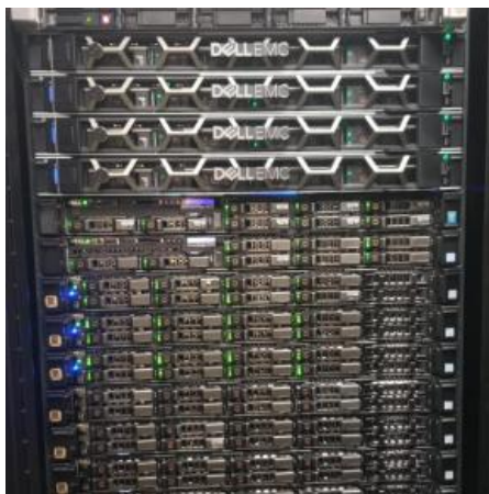
Figure 41: Rack server at NCSR D hosting VMs and network function.
