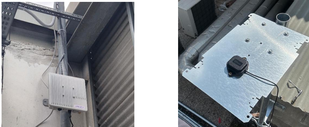
Figure 7: Italian Living Lab – deployed RU and GNSS antenna.
