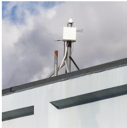
Figure 40: Outdoor Ericsson Baseband 6630 & IRU 8848 unit.
