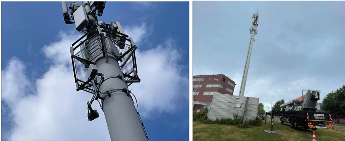
Figure 18: gNodeB in the Dutch trial site.
