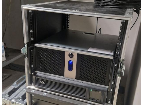
Figure 6: Italian Living Lab – deployed gNB.
