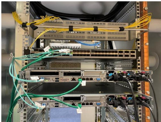
Figure 19: Edge hardware, located at the KPN Metro Core.
